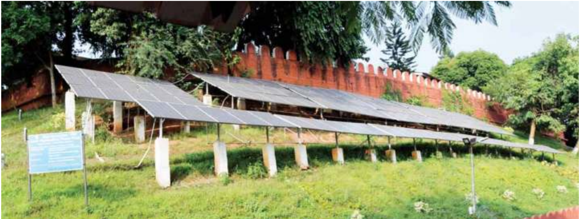
Solar power plant installed at Raj Bhavan
